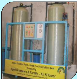
Water Filtration Plant
