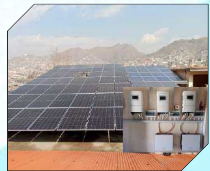
24 KV Solar System
