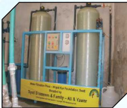
Water Filtration Plant
