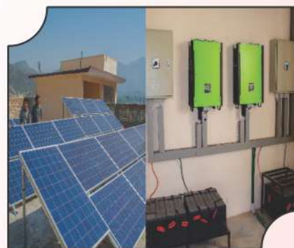
20 KV Solar System
