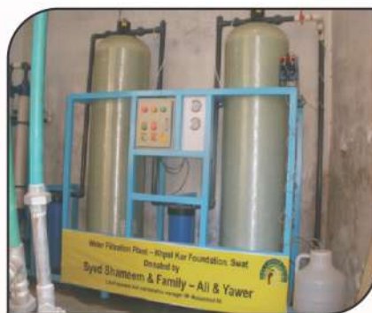
Water Filtration Plant
