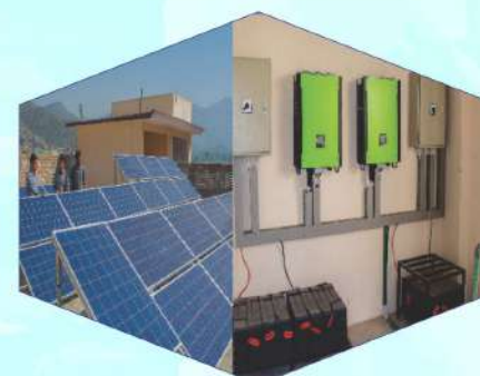
20 KW Solar System
