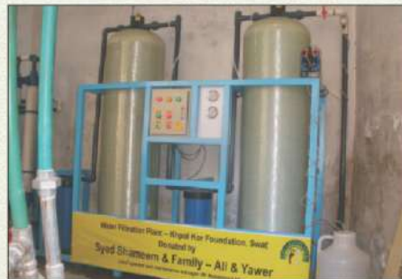
Water Filtration Plant
