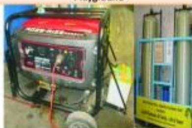
Generator/Water Filtration Plant
