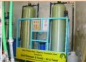
Water Filtration Plant
